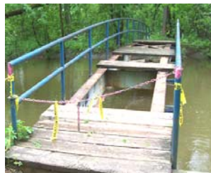
Vandals destroyed planking on the bridge leading to the Ellsworth section this spring. It's been repaired by Wayne County Parks. But a repaired bridge means other potential problems. See page 5.
