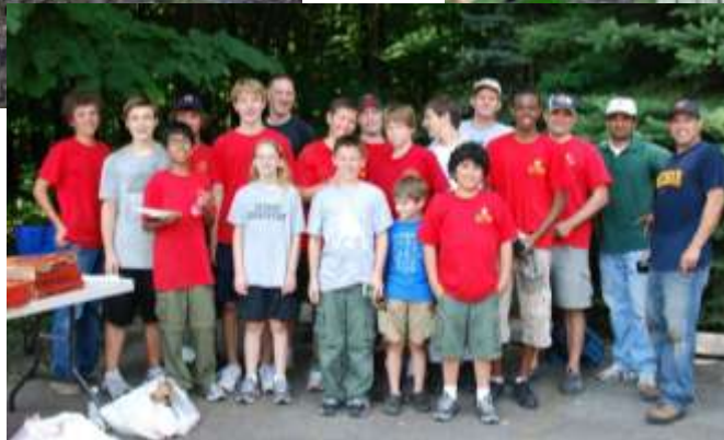
James Obermaier, Troop 1032, North Star Unit, and his team built boardwalk on Tulip Trail in July. James (upper-left) stands on the trail BEFORE. (Upper-right) the new boardwalk. The bottom photo is the team. Wayne County Parks and HNPA thank them for a great job. HNPA provided a small amount of financial support - thank you, members.
