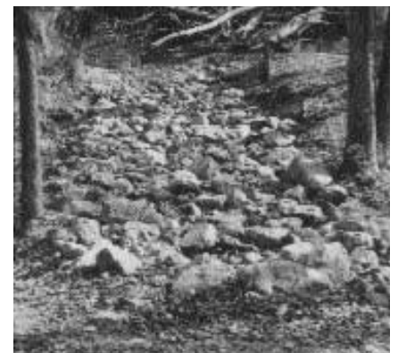
Area after repairs. Eroded areas have been filled in and a spillway (the rocks) added. Whether it will be effective in the long term is not yet known but HNPA will continue to monitor it.
